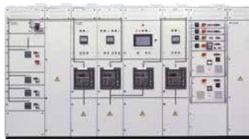
ASSOL LV SWITCHGEAR WITH AN MONITORING AND DIAGNOSTIC SYSTEM LOCAL VISUALIZATION PANEL
